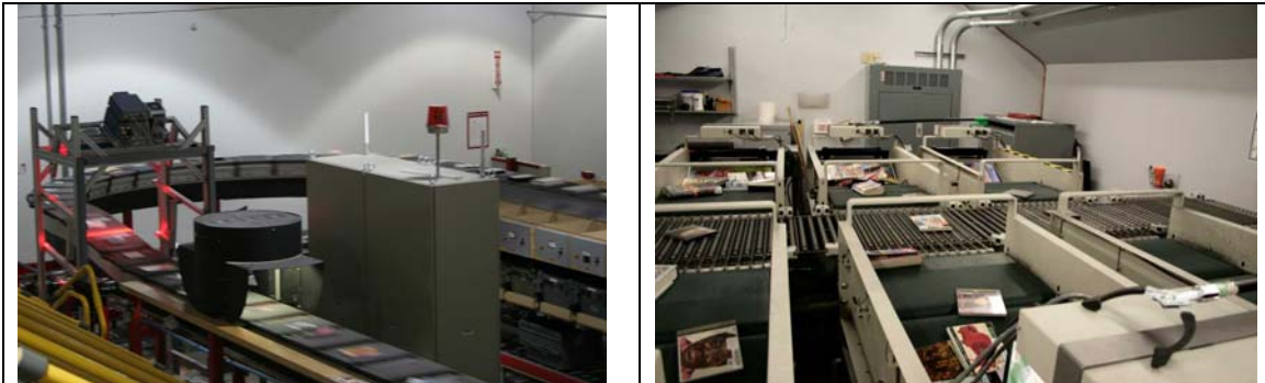
Figure 4: Automated Material Handling System from King County, WA
